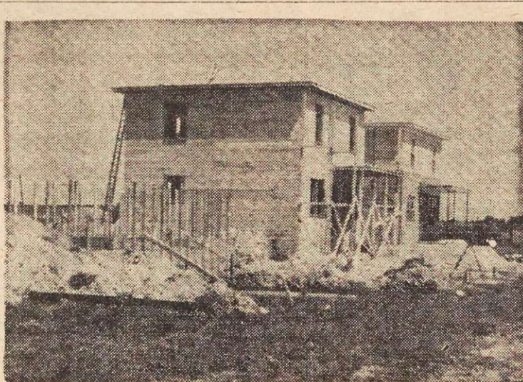
10 homes like this ones are being built at Joliette and sold for 6000 dollars to work ers.
